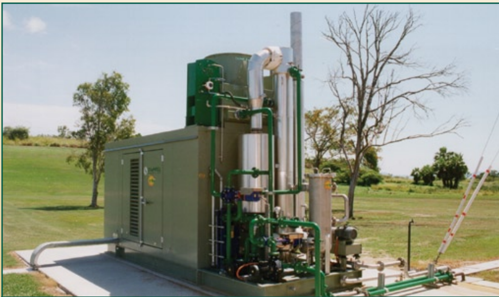
Biogas Cogeneration Plant at Mount Saint John wastewater treatment facility
